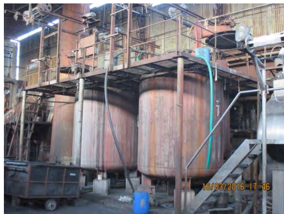
Caption: Thermic-fluid heater at Shree Rajaram Mills
